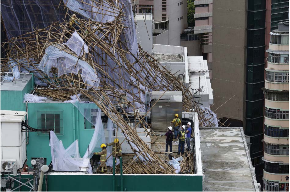
圖 3.3.8 灣仔菲林明道一幢商業大廈外牆一幅棚架倒塌。(相片由中國日報提供) Figure 3.3.8 The scaffolding of a commercial building at Fleming Road in Wan Chai collapsed. (Photo courtesy of China Daily)
