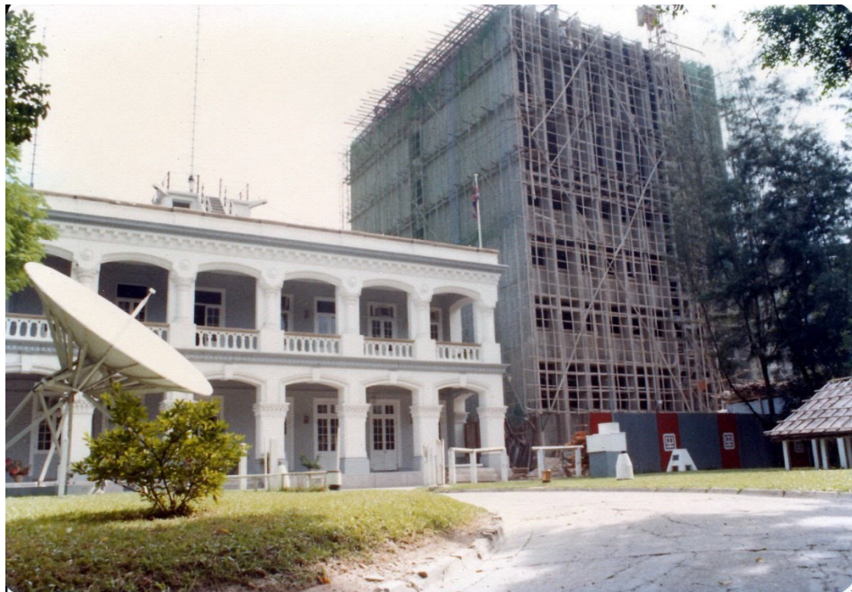
Figure 25. Photo of the Centenary Building under construction in 1980 (Photo courtesy of Dr C M Tam)
