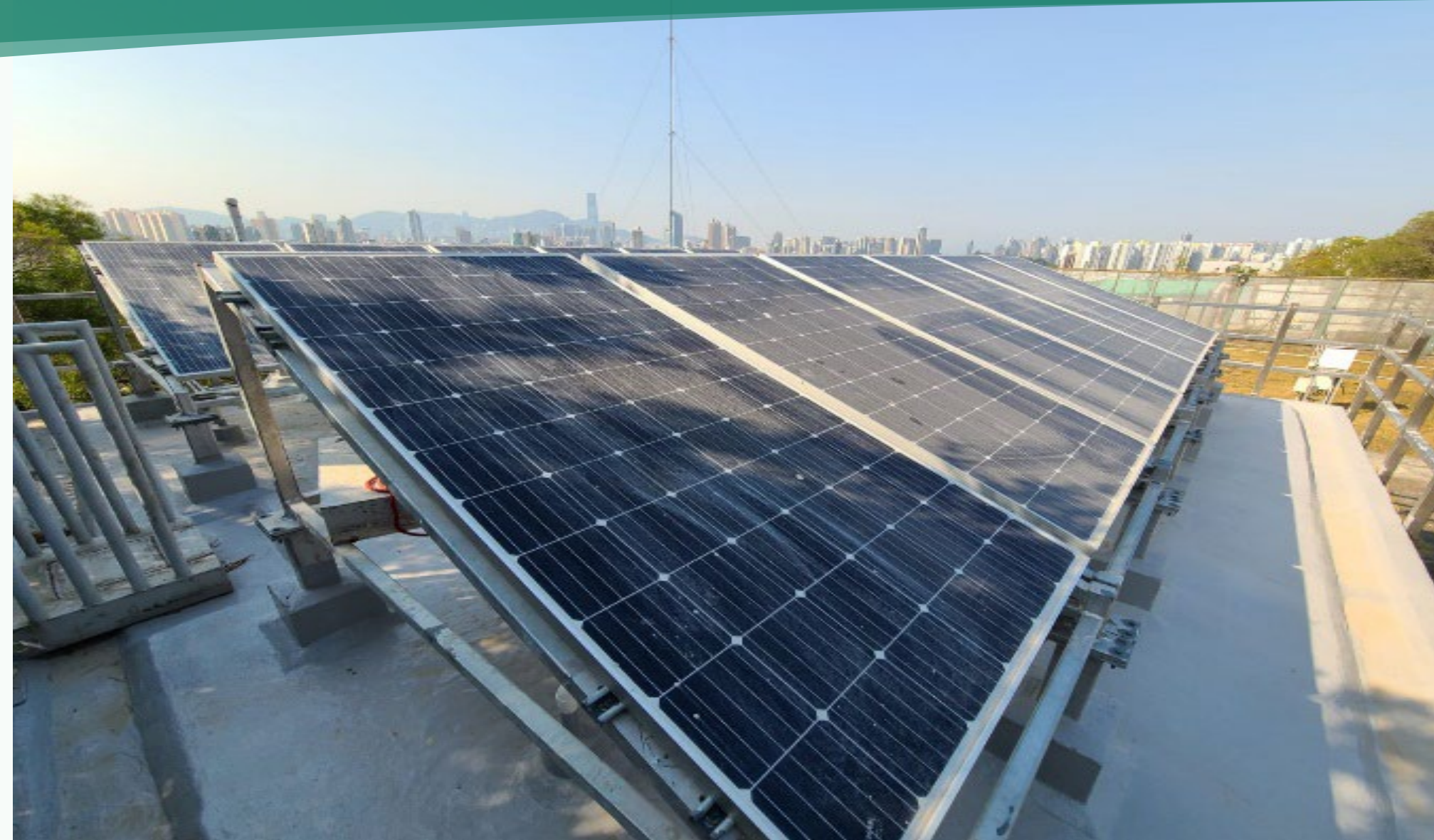
Solar panels in Kowloon Tsai Radar Station
