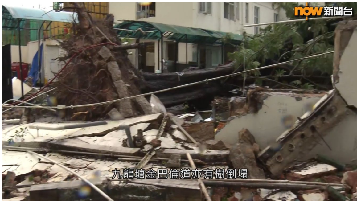
圖 3.11.16 樺加沙襲港期間，九龍塘有獨立屋的外牆被塌樹壓毀。(鳴謝：Now新聞) Figure 3.11.16 During the passage of Ragasa, the wall of a detached house in Kowloon Tong was damaged by a fallen tree. (Courtesy of Now News)
