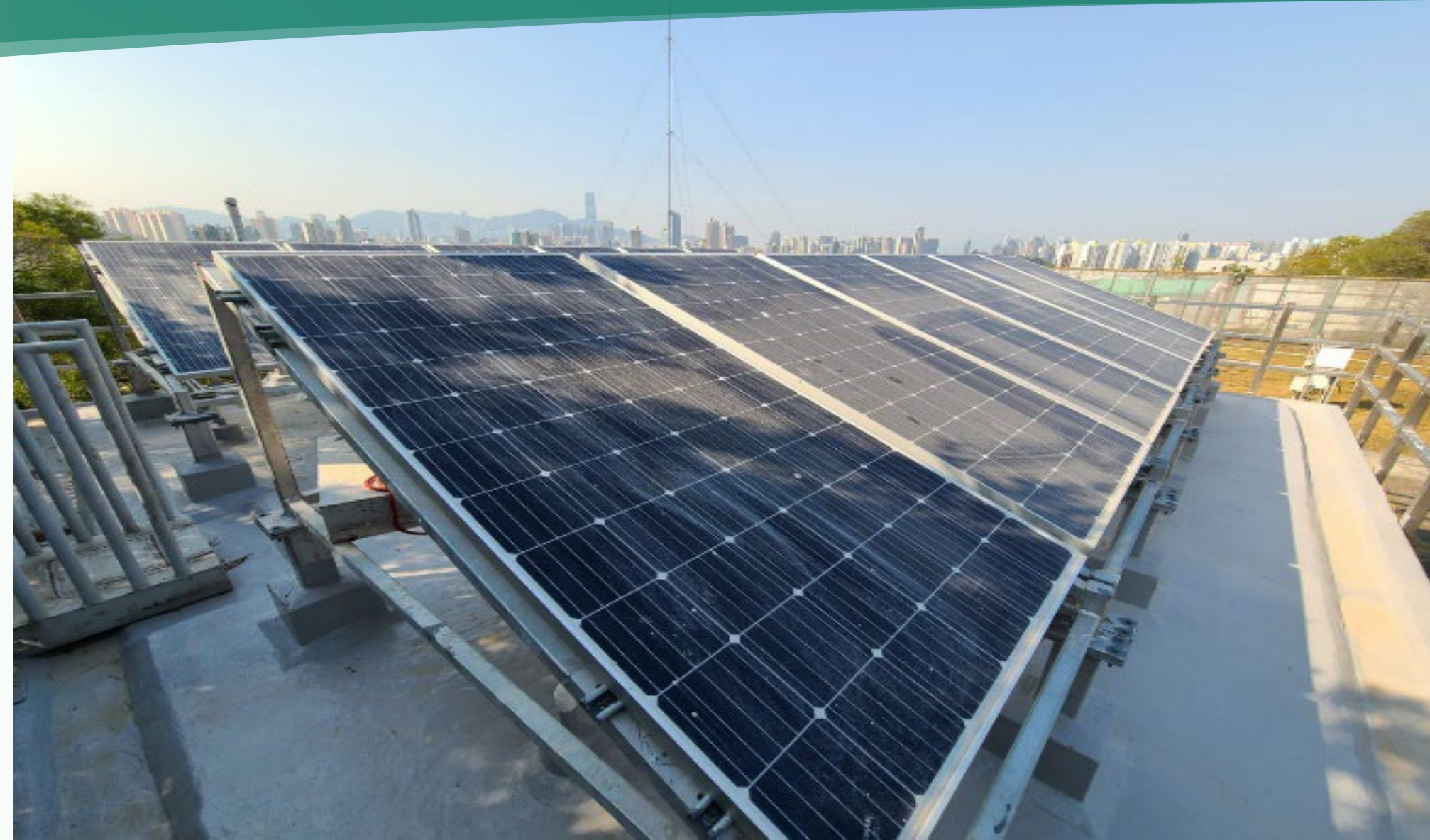
Solar panels in Kowloon Tsai Radar Station
