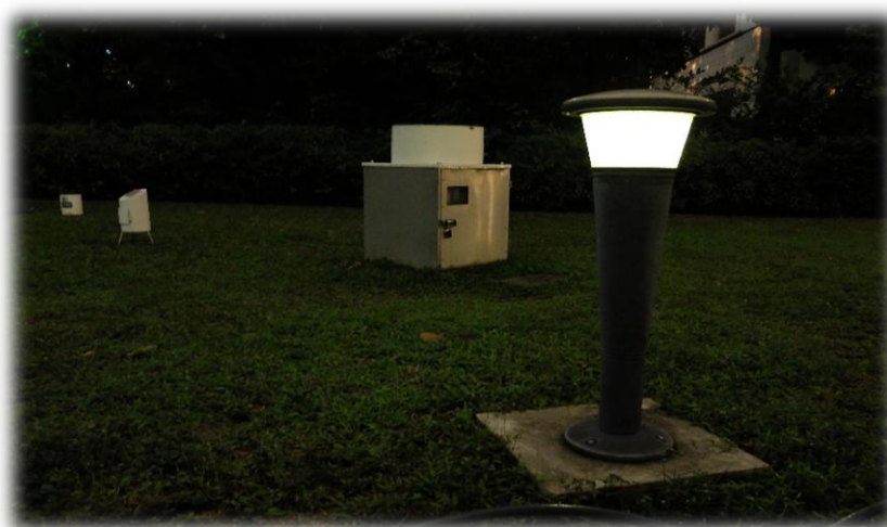
Fig 18: Bollard lamps at HKO HQ using solar power.
