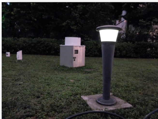
Fig 21: Bollard lamps at HKO HQ using solar power.
